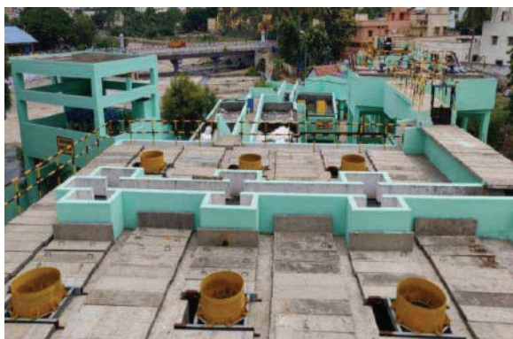
Figure 66: Vellakuttai STP-13 MLD
